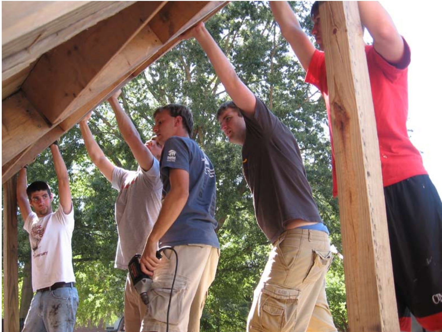
Teamwork: NC State Habitat members and officers Jon Weaver, Ashley Cowan, Matt Poisel, Andy Binder, and David Hoffman hang out under the floor of the Habi-Shack during deconstruction.
